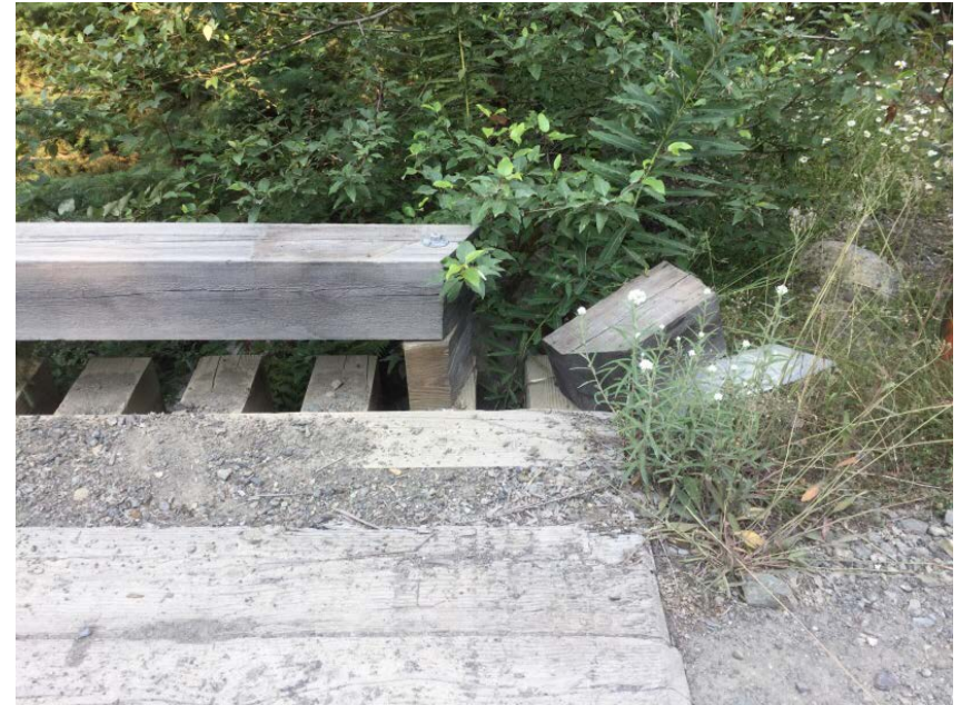
Guardrail and riser damage
